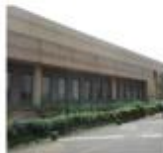
劣化が進む外壁
